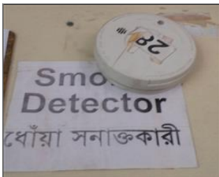
Photo of fire safety equipment F14 Smoke Detector.jpg
