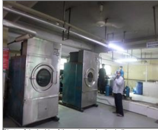
Photo of the inside of the main production hall B12 Wash Section Overview.jpg
