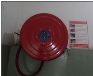
Photo of fire safety equipment F4 Fire Hose Reel.jpg
