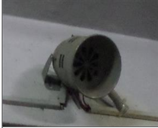
Photo of fire safety equipment F10 Fire Alarm System.jpg
