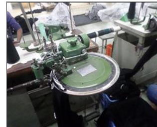
Photo of non-conformity Linking machine guards missing.jpg
