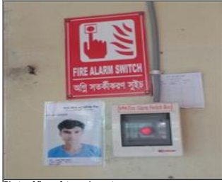
Photo of fire safety equipment F6 Fire Alarm Switch.jpg
