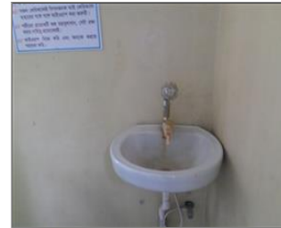
Photo of non-conformity Spot removing room - inappropriate eye wash station.jpg
