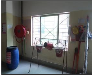
Photo of fire safety equipment F1 Fire Fighting Equipments.jpg
