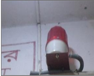
Photo of fire safety equipment F11 Visual Fire Alarm System.jpg
