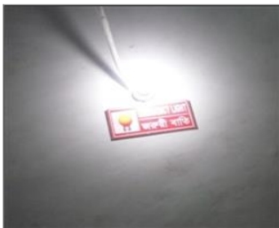
Photo of fire safety equipment F9 Emergency Light.jpg
