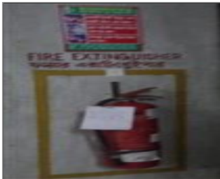
Photo of fire safety equipment F3 Fire Extinguisher.jpg
