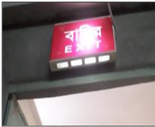
Photo of fire safety equipment F8 Exit Sign.jpg
