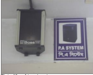
Photo of fire safety equipment F5 PA System.jpg
