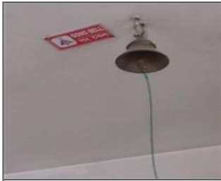
Photo of fire safety equipment F7 Gong Bell.jpg
